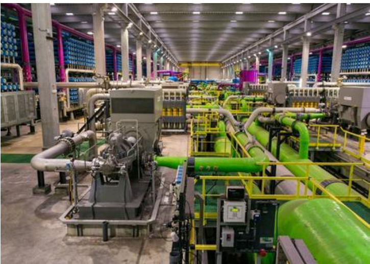
Desalination plant of Llobregat (Aguas Ter Llobregat)
